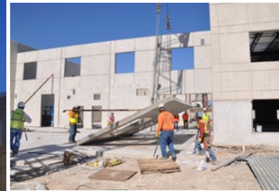
Balfour Beatty recently completed the Round Rock ISD, Joe Lee Johnson Elementary School, a 118,324 SF tilt wall school with 48 classrooms, administrative spaces, library, two music rooms, two art rooms, a cafeteria dining area, and a gym.
